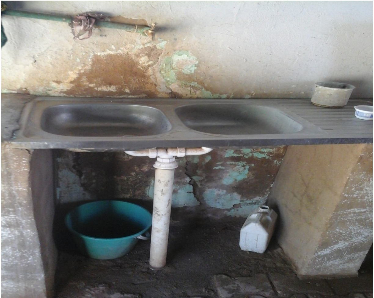
Plate (3): Cracked floor and wall in addition to dirty fixed installed wash basin for utensils in the hospital kitchen
